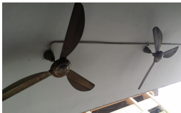
Figure 3.4.4.3.3: There are 2 ceiling fan in Room 3 but they are turned off at the time of the reading as this outdoor seating area is less preferable.
