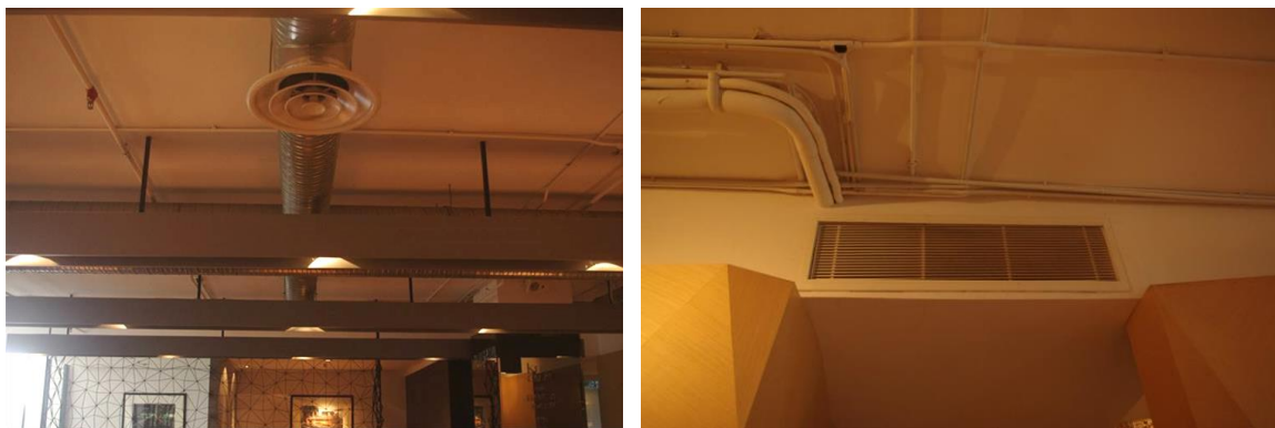
Figure 3.4.4.4.6: Circular and rectangular diffusers are found in the main dining area.
