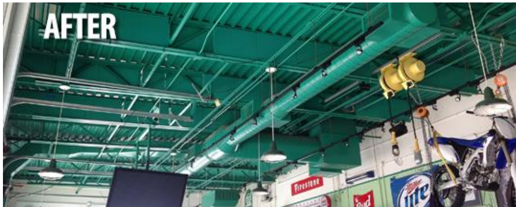
Figure 3.1.1.6: Custom coated Eco-C-Tex to match the ceiling was hidden within trusses to prevent disturbing the ceiling’s unique look. (Source: Soundproofing a Restaurant Case Study: Quaker Steak & Lube, 2014)
