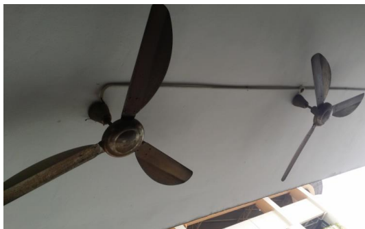
Figure 3.3.1.2.3: Ceiling fan found in the outdoor seating area, Room 3.
