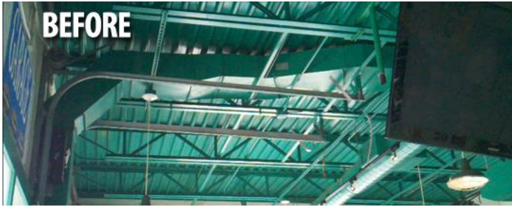
Figure 3.1.1.5: Restaurant noises became unbearable when they reverberated in the unusually high, metal ceilings. (Source: Soundproofing a Restaurant Case Study: Quaker Steak & Lube, 2014)
