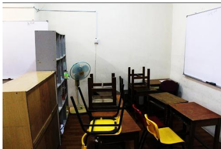
Figure 2 Improper partitioning of spaces.
