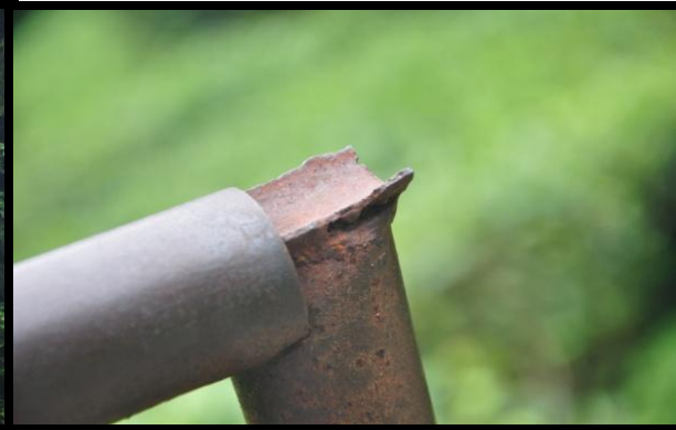
RUSTING OF STEEL
