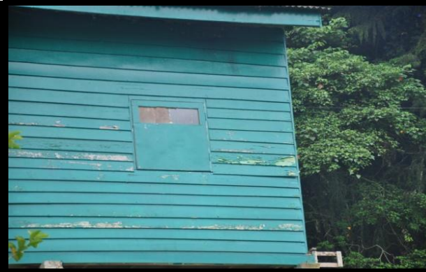
PAINT PEELING OFF
